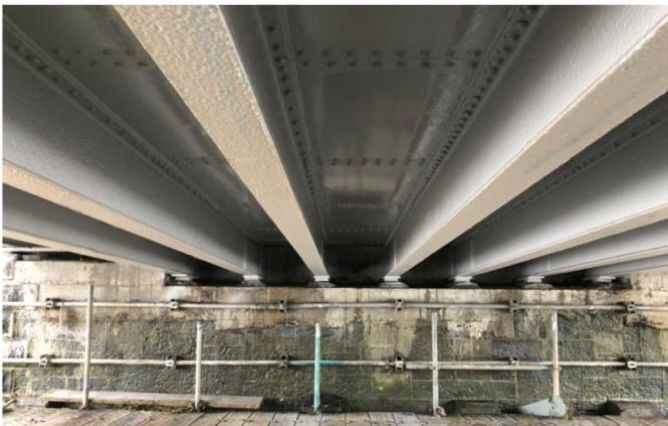
Span 4, two coats of paint have been applied and new bearing bds replaced
